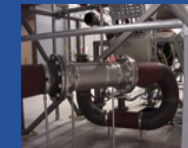
Bleed System & Auxiliary Power Unit
