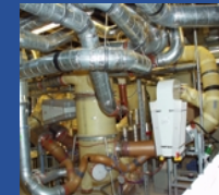
Air Generation & Mixing
